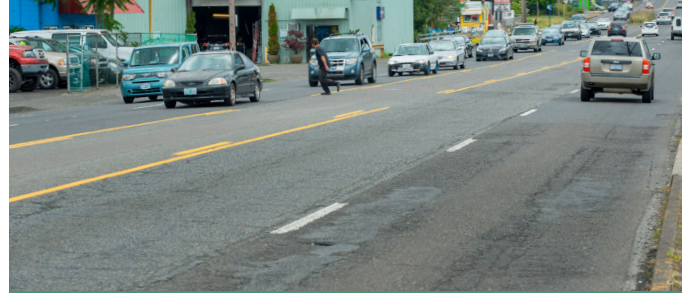
Existing roadway in need of repair and upgrades on SE 82nd Avenue in the project corridor.
